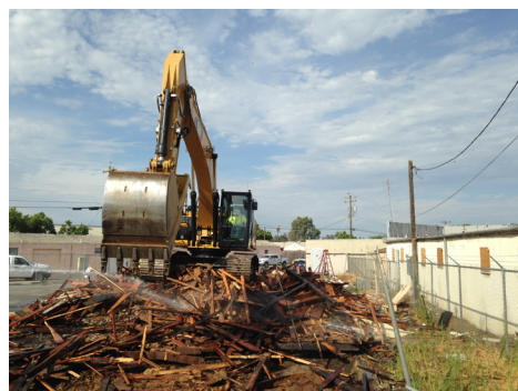
J. Kroeker, Inc. demolishing the Hollywood Inn in downtown Fresno on July 14.
