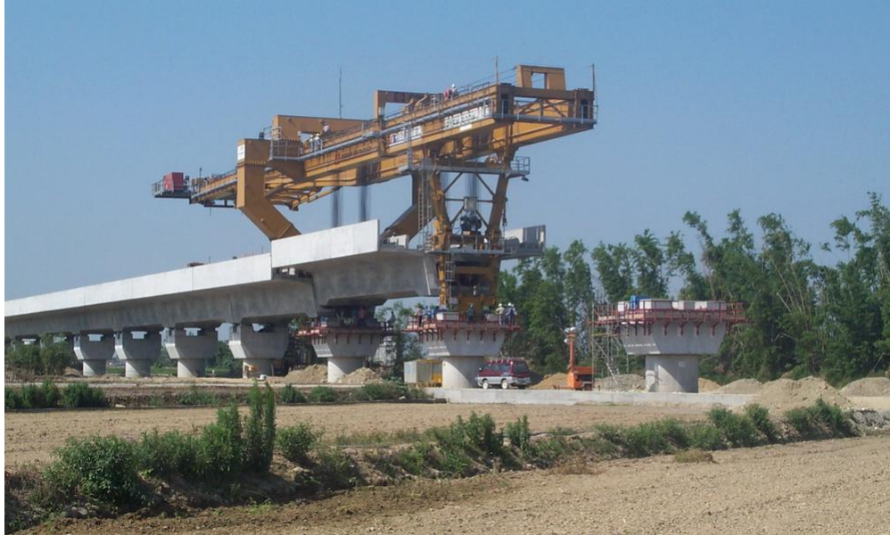
Figure 6-4: Example of Overhead Gantry
