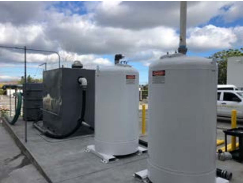
SVE blower and carbon filter vessels.
