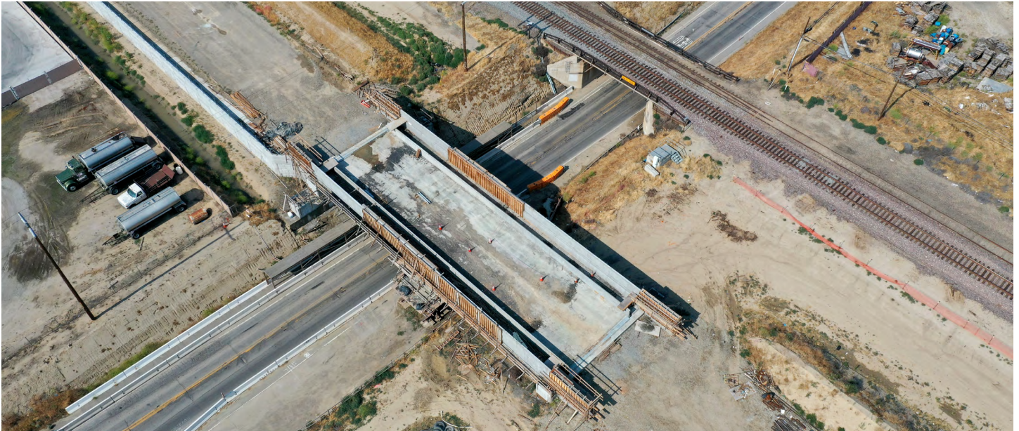
The grant will rebuild the existing freight grade separation at the top right to accommodate four lanes of traffic underneath and a sidewalk, in addition to other improvements.
