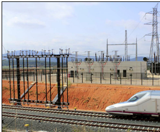
Figure 2-25 Traction Power Substation
