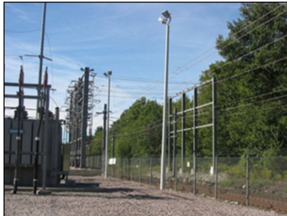
Figure 2-29 Paralleling Station Overhead Catenary System Gantries
