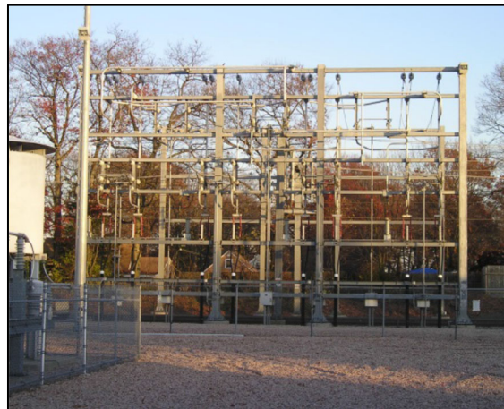
Figure 2-26 Traction Power Substation Overhead Catenary System Gantry
