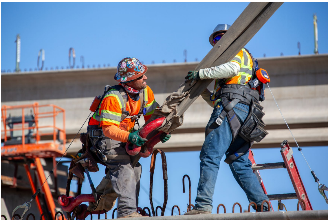
Photo: The Wasco Viaduct in Kern County will take high-speed trains over the existing BNSF freight tracks.
